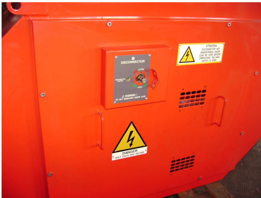
Picture 7 Device detail for internal line disconnector
